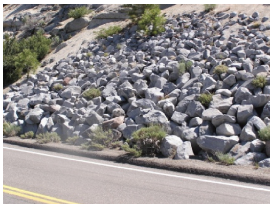
Figure 11: Rock slope protection or ‘rip rap’ can reduce erosion on bare slopes.
